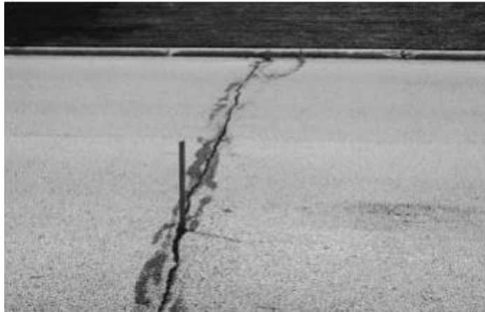
Gambar 3. Retak memanjang/melinang ( Longitudinal and Transverse Cracking ) (Hardiyatmo, 2015)
