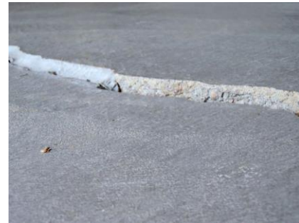
Figure 4. Crack on the floor plate. ( https://www.totalfoundationsolutions.com/foundation-repair/foundation-services/floor-symptoms/floor-cracks/ )
