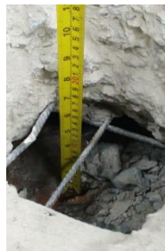
Figure 3. A gap between the ground and the slab. (Located at Sabang)
