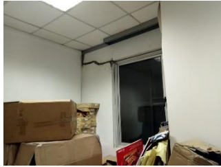
Figure 2. Crack on the wall and ceiling. (Located at Sabang)
